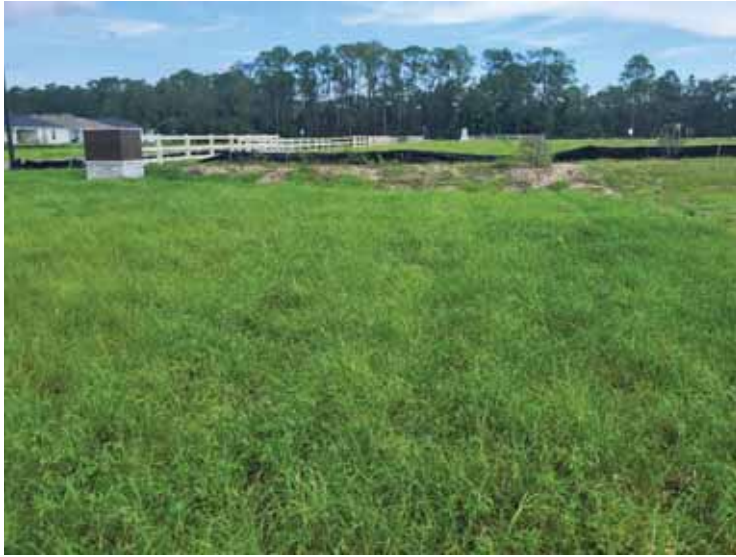
Location 4: Berm lacking turf.
