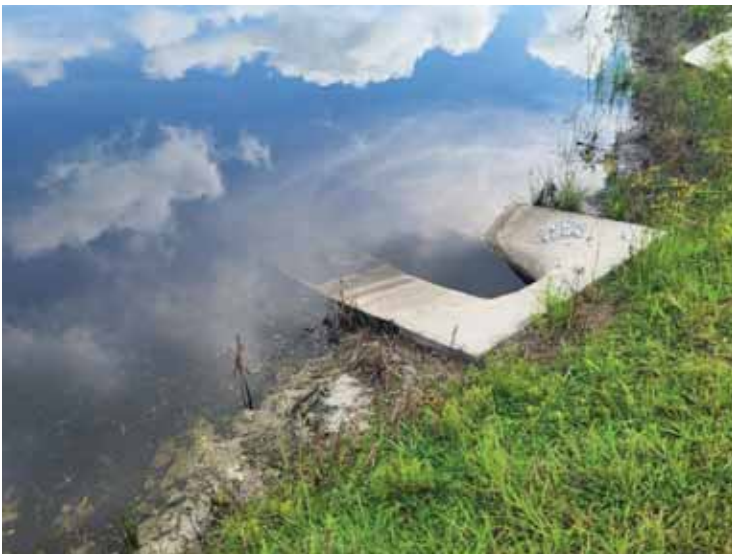
Location 3A: Mitered End Section starting to erosion around the sides.
