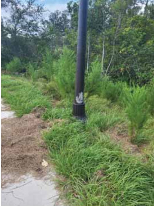
Location 16: Street light pole damage.
