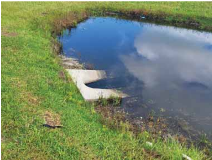
Location 5: Mitered End Section starting to erosion around the sides.
